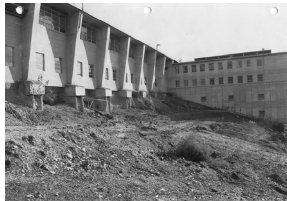
Figure 43. View of erosion at the west side of the Warehouse/Laundry/Annex building prior to construction of the retaining wall, December 6, 1977. Source: GSA Archive, image DC1470SE0P020.
